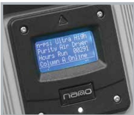
PLC controller with clear text display
